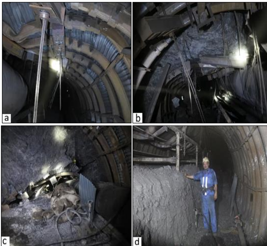
Fig. 1. Examples of squeezing in Slope No. 2, Parvadeh 1 Mine: (a) movement of the roof causing deformation of the steel arches, (b) significant roof movement leading to severe deformation of the steel arches, (c) extreme roof movement resulting in almost complete closure of the tunnel, and (d) substantial heaving of the floor
